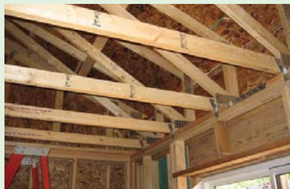
An example of energy savings built into a new home: Raised heel roof trusses that extend the top of exterior walls allow for a uniformly thick layer of insulation. Ordinary roof trusses that come to a point at the exterior wall do not allow for thick insulation layers on the sides, resulting in energy losses over the lifetime of the house. Photo source: National Renewable Energy Laboratory.
